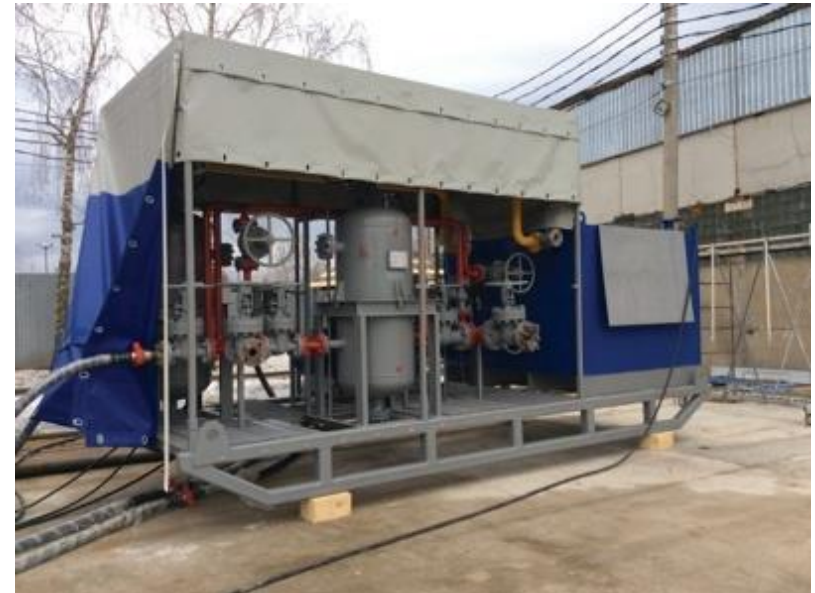
Power block of MPU
